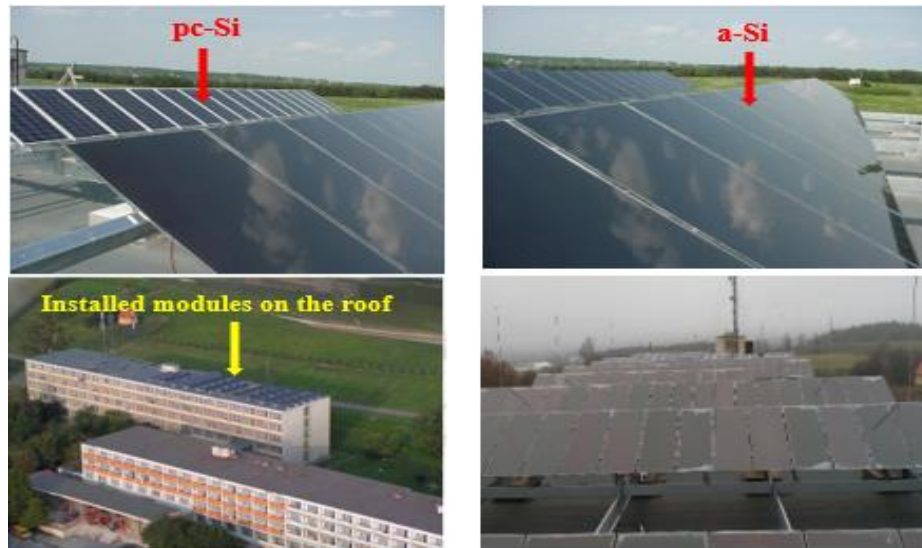
Fig. 3.7. Installed PV array
